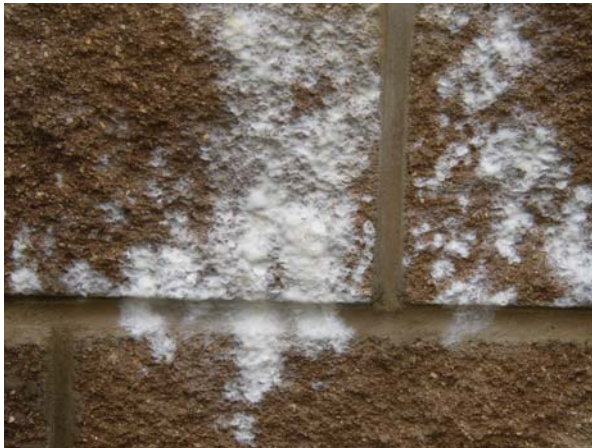
An example of efflorescence caused by calcium chloride in concrete.
